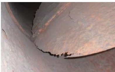
Wasted fire damper flap
