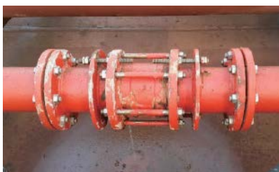
Leaked fire line
