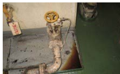
Oil leakage and accumulation
