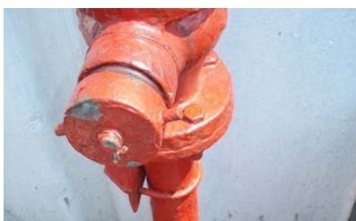
Leaked fire line
